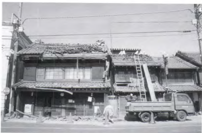
Right after the earthquake / 被災直後
