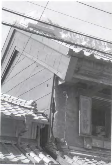
Damage to main ridge and earthen walls 棟、外壁に被害
