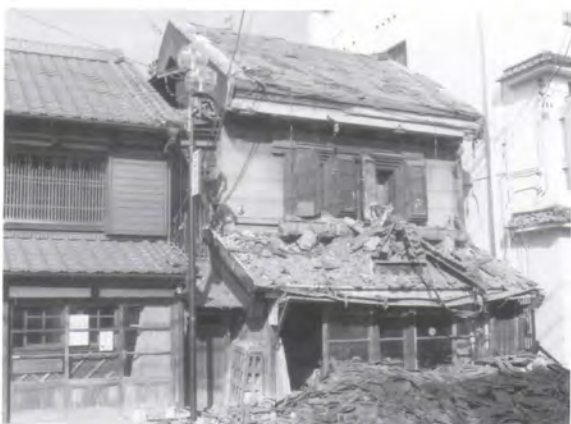
Right after the earthquake / 被災直後
