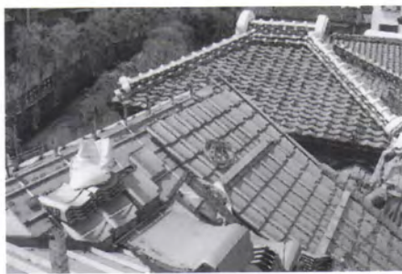
Damage to store roof / 店舗屋根修理
