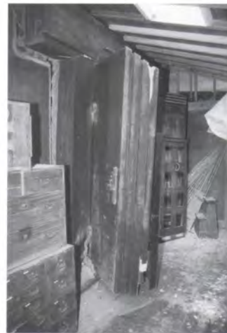
Damage to storehouse earthen doors 土蔵観音開き扉被害
