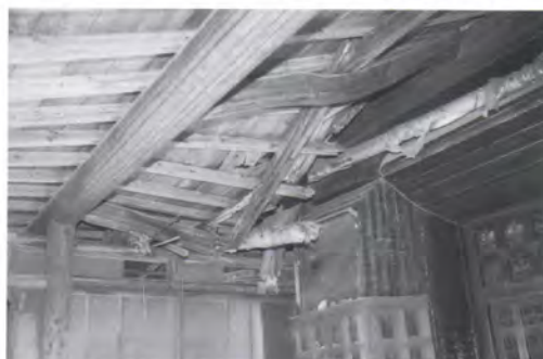
Storehouse, damaged lean-to / 土蔵下屋破損
