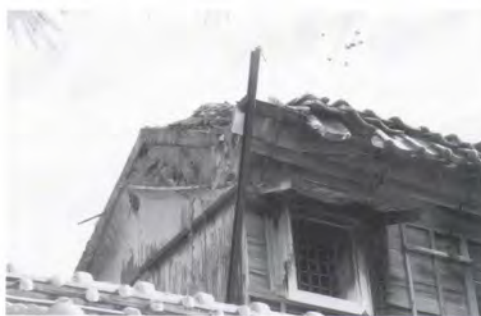
Damage to the earthen-walled storehouse 土蔵の被害
