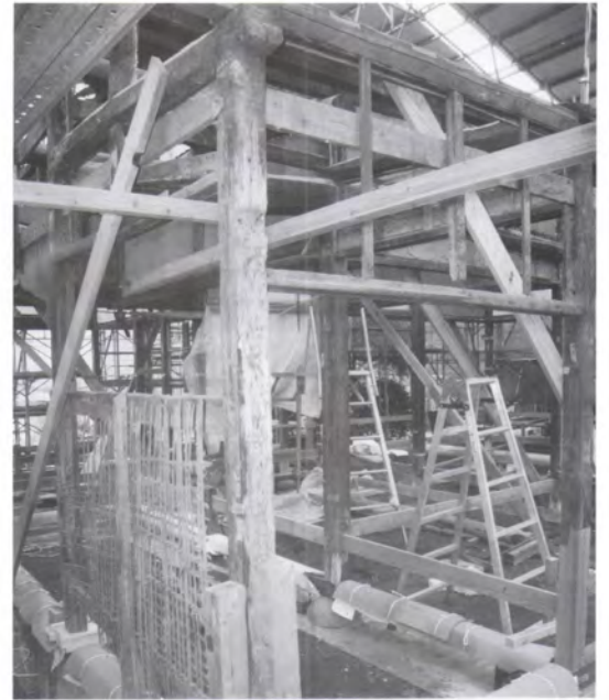
Restoration of the Former Inoh Tadataka Residence reception room / 伊能忠敬旧宅書院修理
