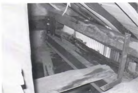
Damage to store roof structure 店舗小屋組被害
