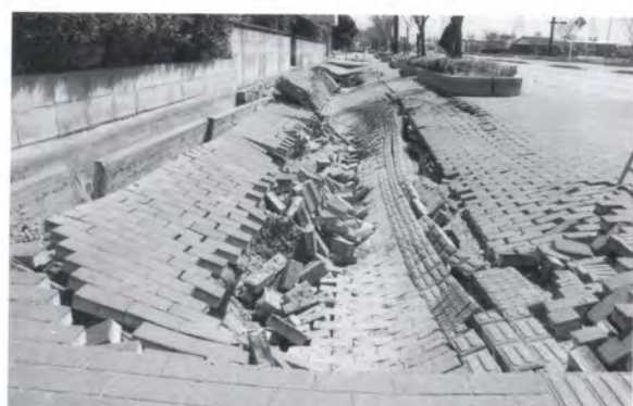
Damage due to liquefaction
