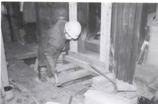
Doors were jacked up and reinforced with a frame ジャッキアップして補助枠
