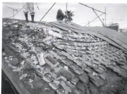
Damage to roof tiles / 屋根瓦の被害
