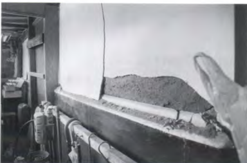
Plaster delamination / 漆喰が剥落
