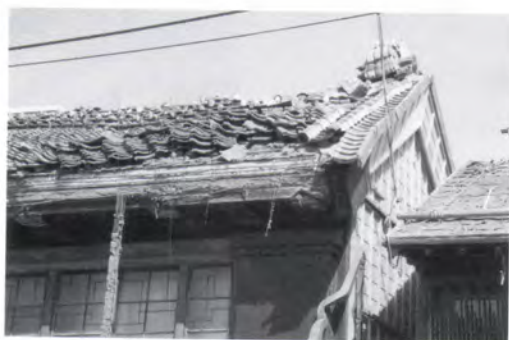
Damage to store roof / 店舗屋根被害
