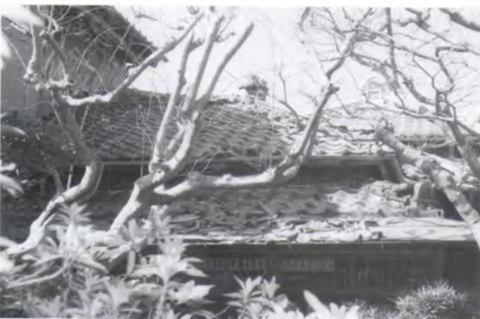
Damage to reception room roof / 奥座敷屋根被害
