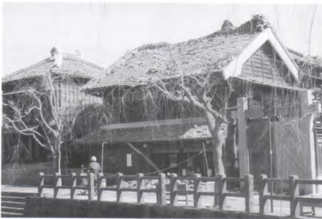
Right after the earthquake / 被災直後
